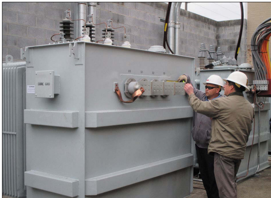
Sylacauga Utilities Board Electric Superintendent Eric Carithers and lineman Jeff Whaley inspect the third transformer.
