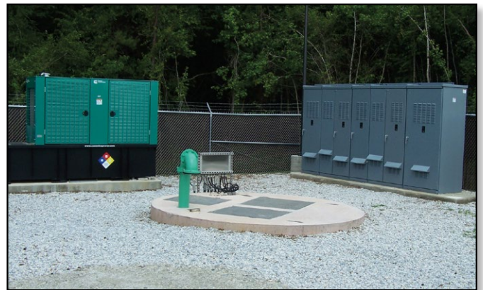
New lift station
