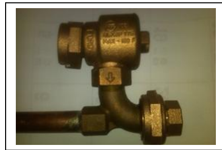
Enlarged Image-Backflow Preventer
