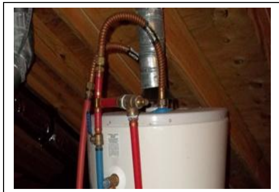
Enlargement of a Retrofit High Temp. Blow-off Valve
